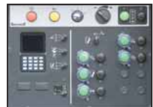
Main control panel
